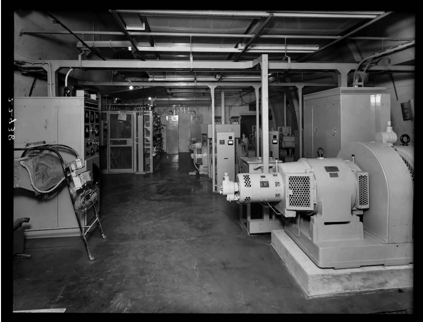
Figure VE 3.8 Plant room with equipment for ventilation and cooling, 1959. Source: BT Archives, ref. TCB417/e22938.
