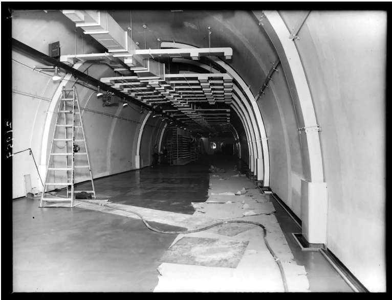
Figure VE 3.3 Upper floor of main tunnel being fitted out with racking to support telecommunication equipment, 1957.
