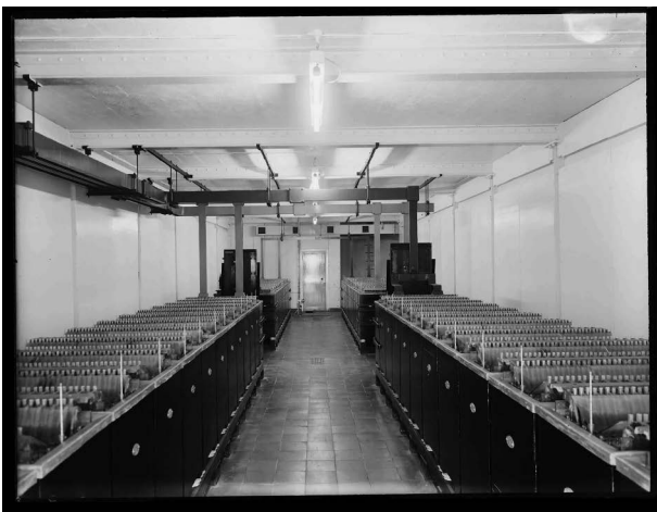
Figure VE 3.7 View of banks of batteries to provide emergency backup power before the diesel generators start-up, 1959.
