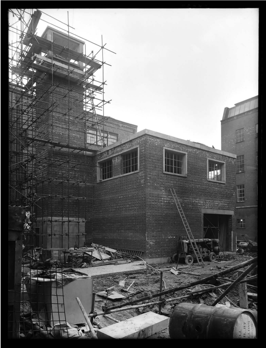
Figure VE 3.5 Completing the utilitarian surface building and ventilation tower at George Street, December 1956.
