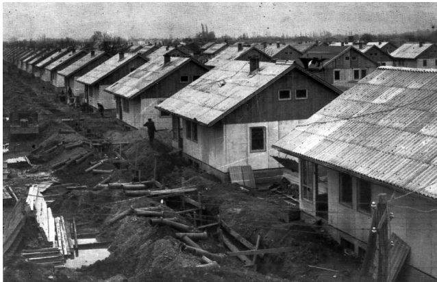
Figure 7.3 Finishing work on the prefabricated houses of the “Taftalidze” neighbourhood. Still existing today, these houses were donated by the government of Czechoslovak Socialist Republic.
