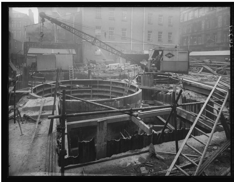
Figure VE 3.4 Completion of the shaft head no. 6 at George Street which would provide the main access to the exchange, March 1960.
